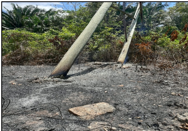
Figure 1 Burnt heel of transmission line structure caused by bush fire in Maskall Village
